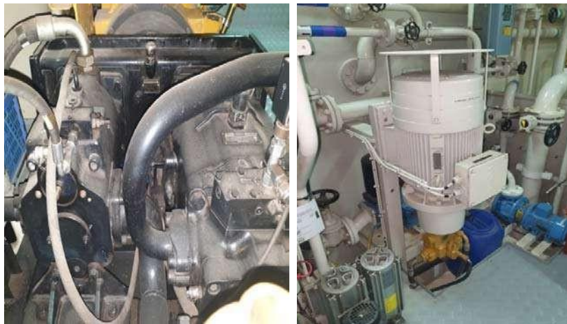
Gambar 3.4 Hydraulic Pump Dan Emergency Hydraulic Pump
